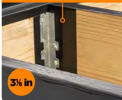
BETWEEN FRAMING AND JOIST HANGERS
